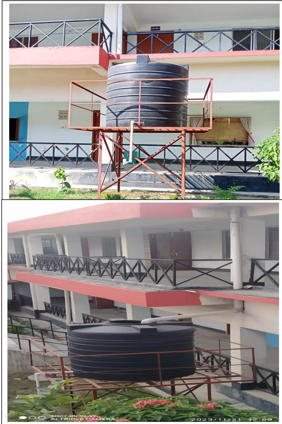
Pipeline system of Rain-water harvesting
